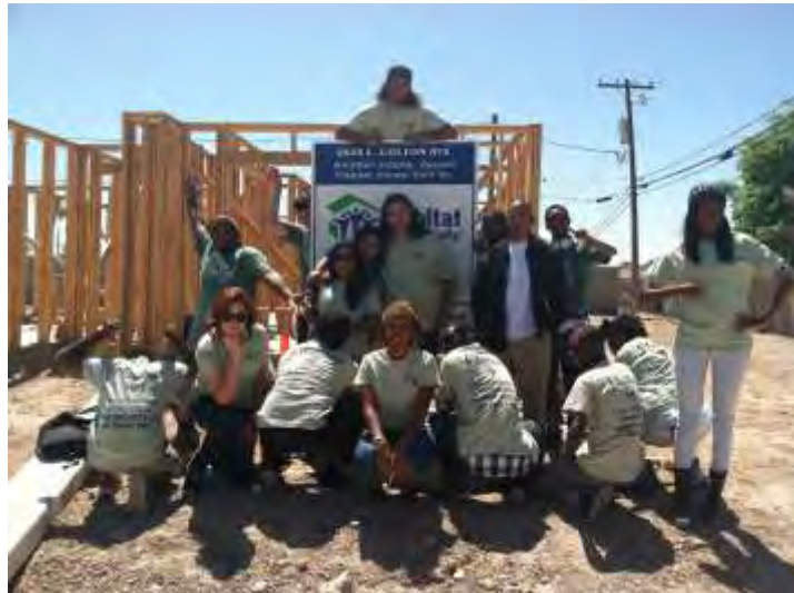
Youthbuild participants get hands on experience and the opportunity to learn about construction.
